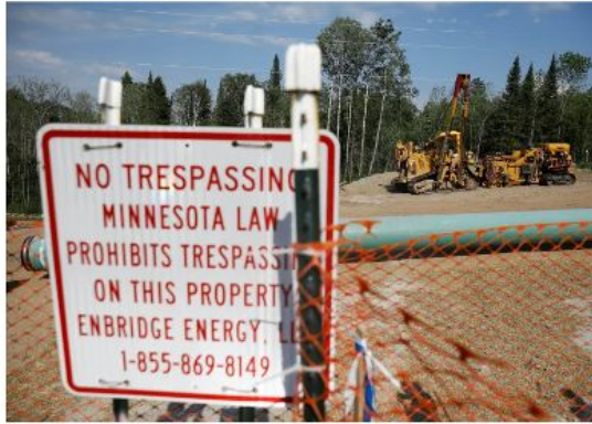
The Enbridge Line 3 pipeline is pictured in place to be buried near Park Rapids on the second day of the Treaty People Gathering, an organized protest of the Line 3 pipeline, built by Enbridge Energy, in Park Rapids, Minnesota, June 8, 2021. (Nicholas Ploss/Reuters)
