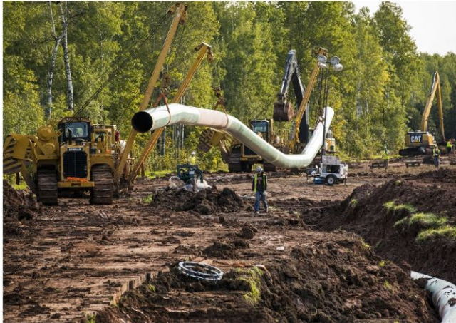
Construction vehicles transport a new section of pipeline to where it will be placed in the ground in September 2017 south of Superior, Wis., as part of the Enbridge Line 3 replacement project. Derek Montgomery for MPR News 2017
