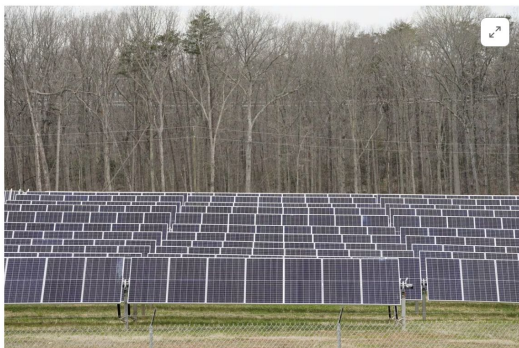
[1/32] Solar panels facing the sun are seen in the Spotsylvania Solar Energy Center, the largest solar project east of the Rockies, in Locust Grove, Virginia, U.S. April 4, 2022. REUTERS/Kevin Lamarque Acquire Licensing Rights
