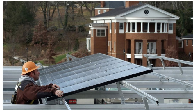
A worker installs solar panels at Washington and Lee University. (Photo courtesy of Secure Futures LLC.)
